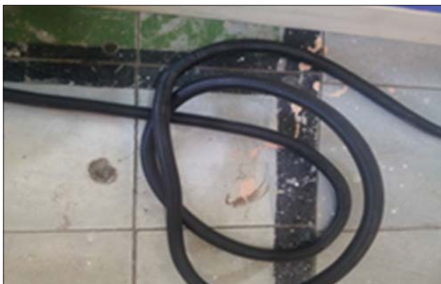
Figure 7: illustrates the cover that contains the wires inside it.
