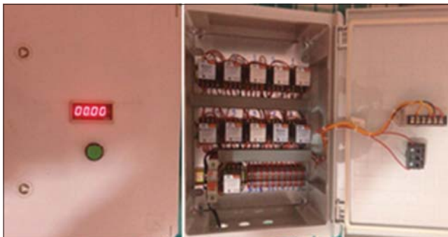
Figure 6: Illustrates the control board and the counter.
